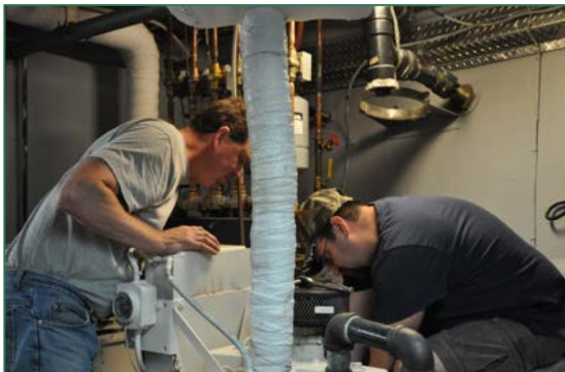
Carl Hatch and Scott Reid completing maintenance checks in the engine room.
